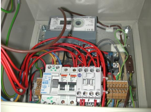
Fig. 9 Energy consumption meter
