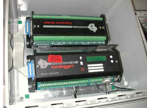
Fig. 10 Data logger (lower) and channel expansion module (top)
